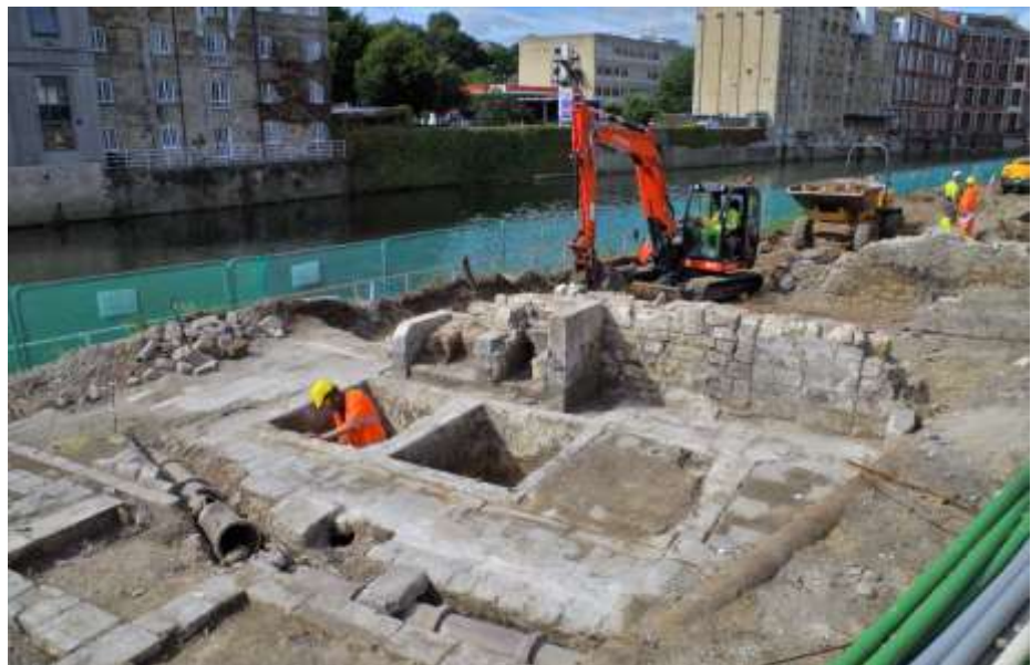
Stone-lined liming pits within a fellmonger's yard and parchment works at 3 New Quay, constructed c. 1775
